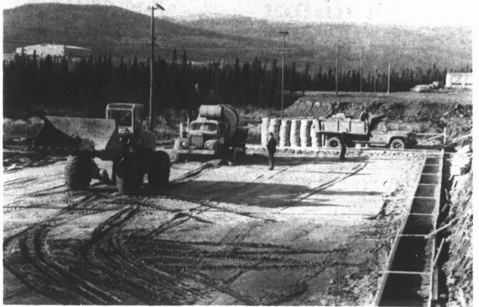
Rapid progress is being made on the construction of the Caro-Wabush Co-op Society building.
